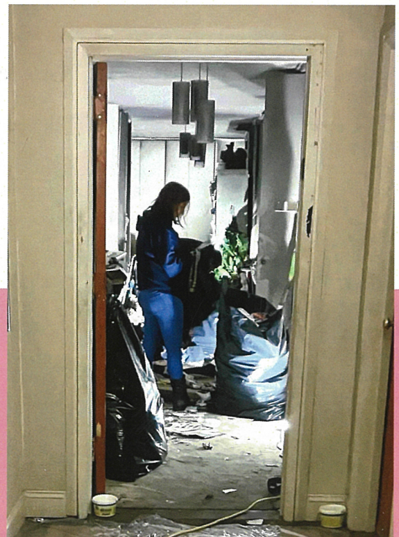
Cleaning up after the fire in unit 14B35. PHOTO: SALLY DOWNEY
